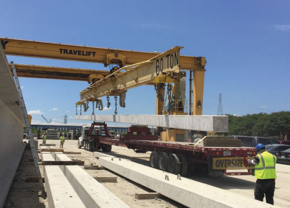
Once a precast concrete pile has been cast and removed from its form, it is fully prestressed and can be easily and safely lifted, handled, and transported to the jobsite. Note that at this stage, the entire pile can be fully inspected. Photo: Roy L. Eriksson.
