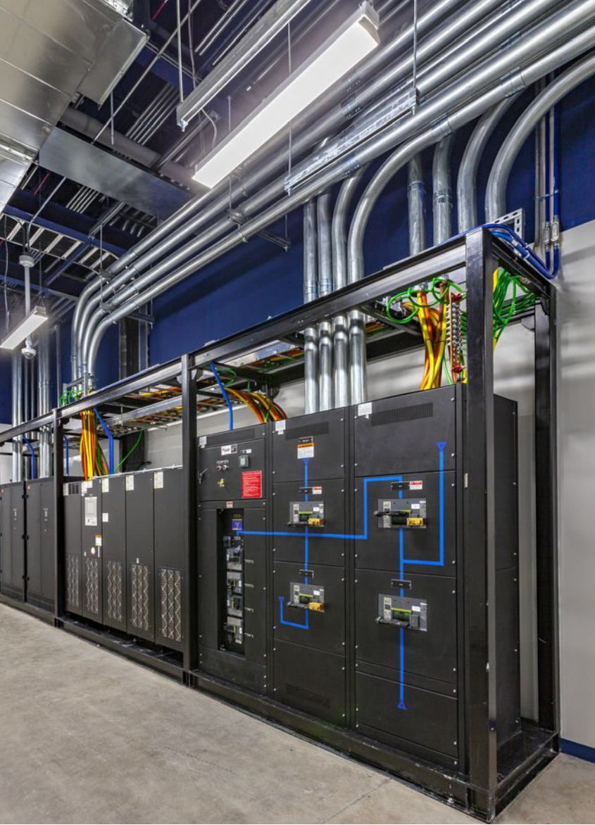
With artificial intelligence, data centers will require larger racks, which in turn requires larger floor-to-floor heights. Photo: HKS/Kevin Perrenoud Photography.
